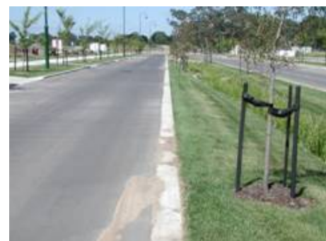
Plate 3-2: Flush Kerb without Setdown, showing Sediment Accumulation on Road
