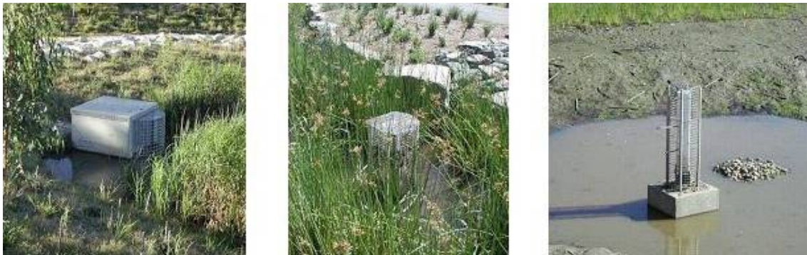
Plate 6-4: Example Outlet Riser Assemblies with Debris Guards
