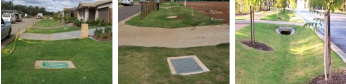
Plate 2-2: At-grade (left) under construction with trees yet to be established, pre-constructed 'at-grade' (centre) and elevated driveway crossings to allow vehicle access across swales
