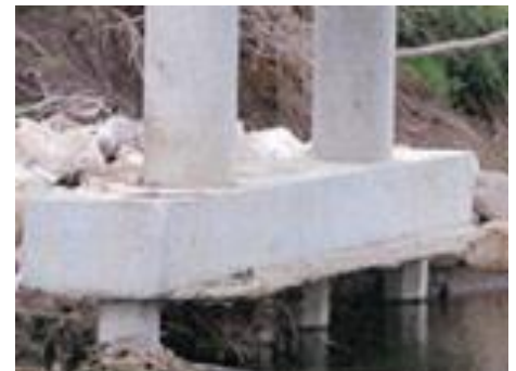
Streambed lowering impacts on structural integrity of man-made assets as well as the stability of streambanks.
